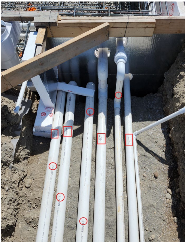
Example of piping back to the equipment room showing pipe sizes and identification of each pipe.
